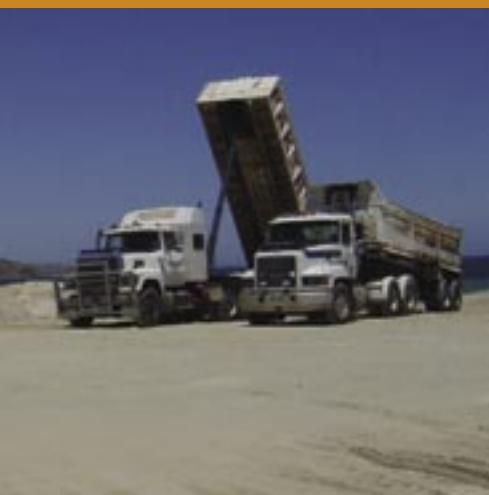
Sand dumping platform at Edwards Street, Brighton – trucks dumping sand on the platform
