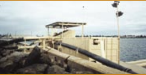
Pipeline booster station operating at Noosa, Queensland (SlurrySystems)
