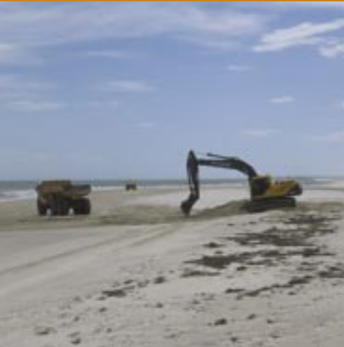
Removing sand from south of the Torrens Outlet, November 2004 (City of Charles Sturt)
