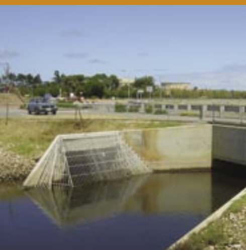
Trash rack covering Patawalonga Creek and Airport Drain entrance into the Barcoo Outlet pipeline
