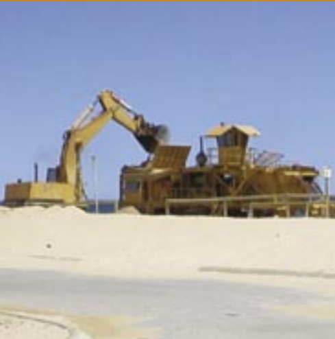
Slurrytrak system in operation at the Dawesville and Mandurah Inlets, Western Australia (CGC Dredging)
