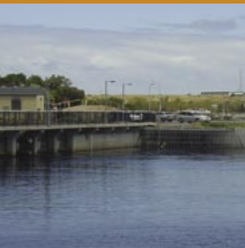
Trash rack covering Patawalonga Lake entrance into the Barcoo Outlet pipeline
